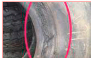
Waterproof Line Crack
